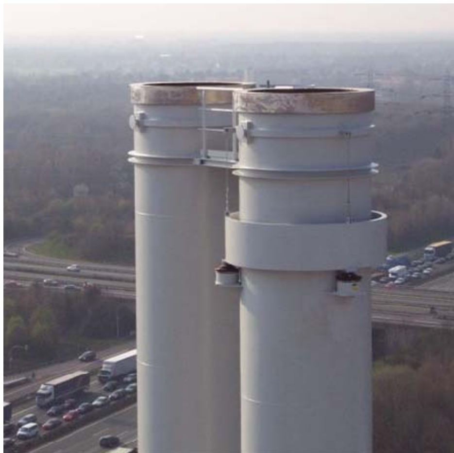
Tuned Mass Damper Ring around a steel chimney
