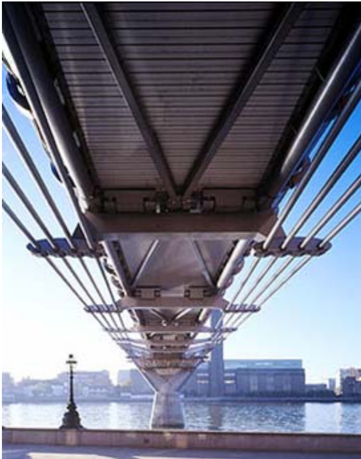
TMDs at the Millenium Bridge London
