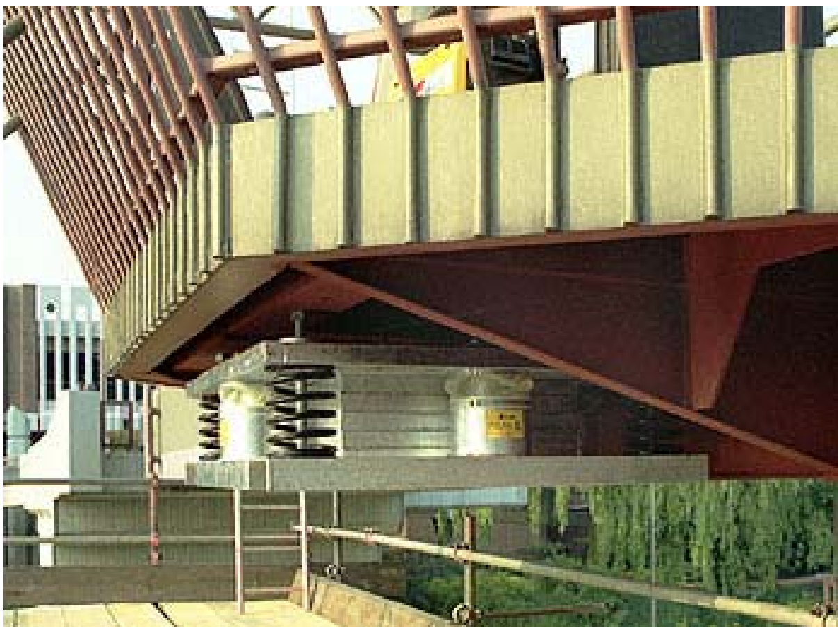
Application of a Tuned Mass Damper at a balcony
